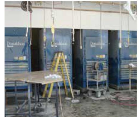
DWS on Granite Finishing 22,000 cfm (37,370 m 3 /h)
