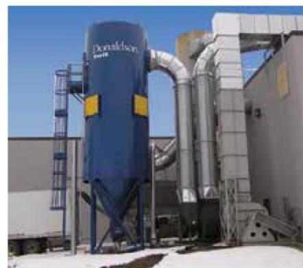
RF - Cabinet Shop 48,500 cfm (82,385 m 3 /h)
