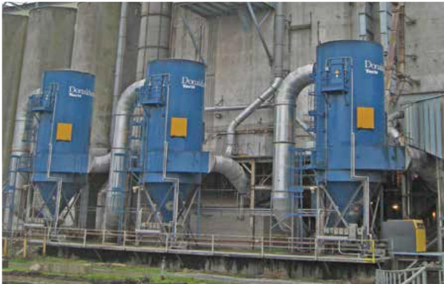
RF - Grain Terminal 61,000 cfm (103,618 m 3 /h)
