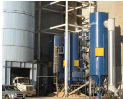
RF - Grain Terminal 34,000 cfm (57,754 m 3 /h)
