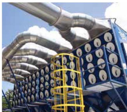
DFO on Sawdust 57,500 cfm (97,692 m 3 /h)
