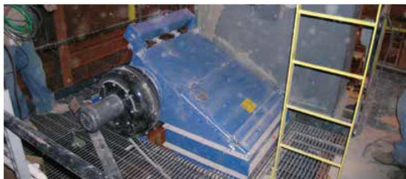
CPV - Bucket Elevator 1,200 cfm (2,038 m 3 /h)
