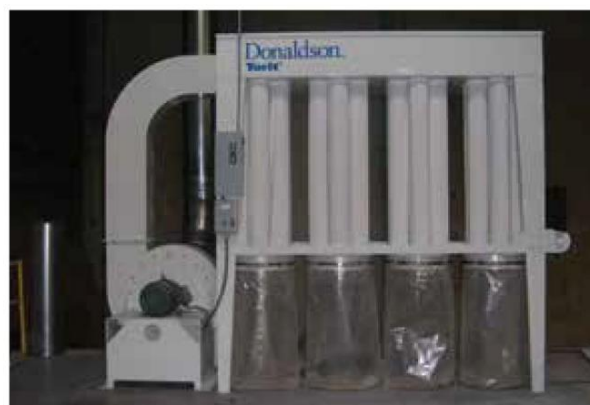
IRD - Wood Shop 5,000 cfm (8,493 m 3 /h)
